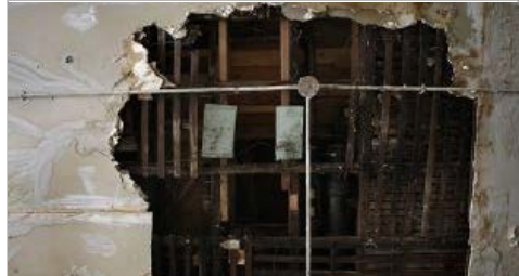
Hotel problems very exposed Residents of SF's All Star Hotel complain of leaks, ceiling holes, floors so slanted people fall down.
